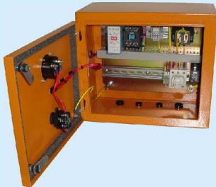
BOREHOLE DOL STARTER
