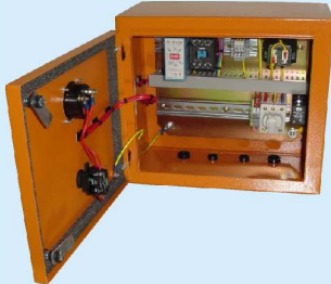
BOREHOLE DOL STARTER
