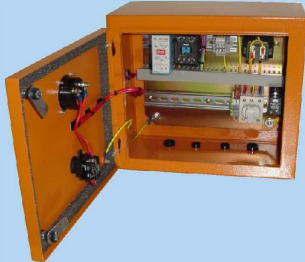
BOREHOLE DOL STARTER
